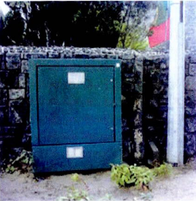
District Regulating Installation (DRI)
